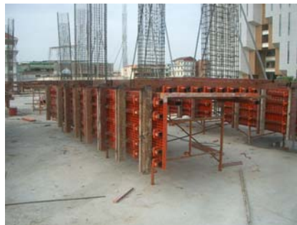
Construction of RC ground floor and columns supporting PT 1 st floor at LCC convention building
