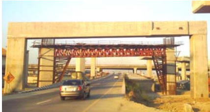
Portal Frame after Tensioning and Grouting while the Scaffolding for the Next Frame
