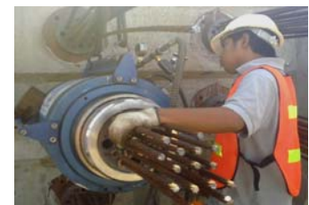
Tensioning of Single Span Frame at 467 ton Stressing Force with 500 ton Stressing Jack
