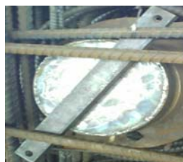
Dead End Anchorage Showing Protection Cap Being Held Temporarily Prior to Fixing with Screw at Cross Bar
