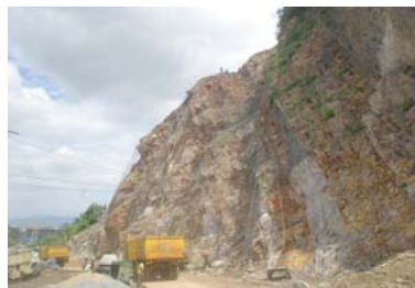
View of Tech9 Scope of protection Works Completed and Road Widening also seen
