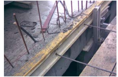
View of PT Slab Edge with Mono Strand Bonded Tendon System
