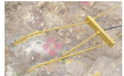
Strands Anchored at Top of Hill to Hard Rocks with Mono Strand Barrel System
